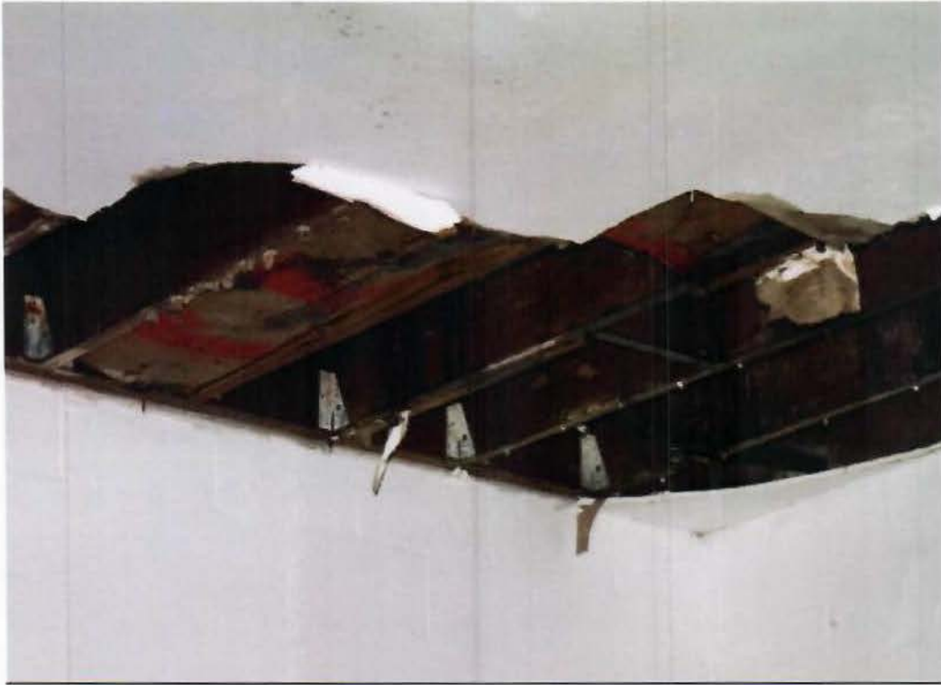
Image #7 shows the roof framing deteriorated wood as well as notched joist
