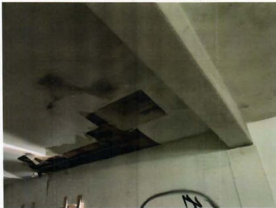
Images #4 shows the concrete beam support the flexible diaphragm and deterioration of the roof framing
