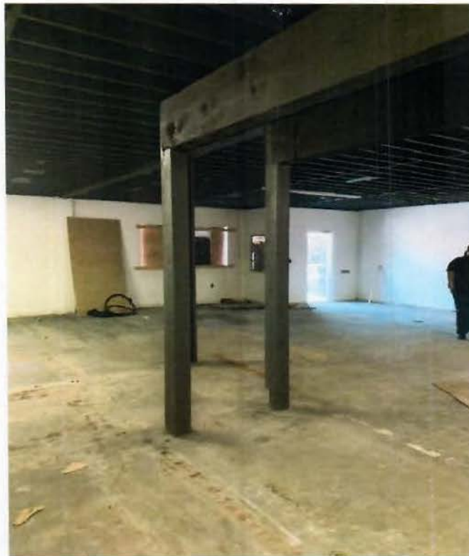
Image #3 shows the floor joist supported with wood beam which support with 2-2x6 stud
